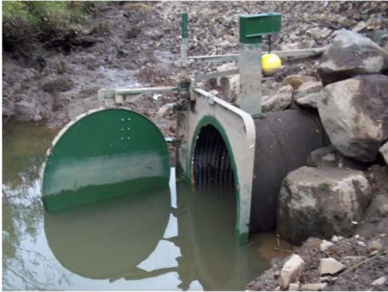
Figure 3. Side-hinged aluminum tidegate door in working location.
