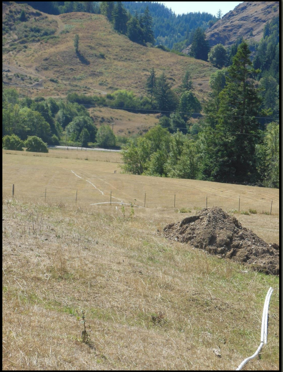
The upper holding tank and view of pipeline looking south to lower site:
