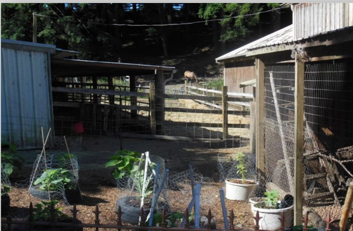
Main Barn, adjacent drainage (facing south). AFTER: Culvert has been installed so that there is no longer any above-ground flow through the stable yard; tree removed and vegetable garden planted (7-3-2018).
